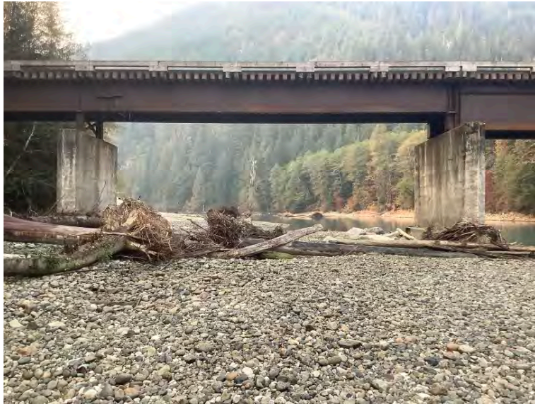
Debris around 2 left bank piers
